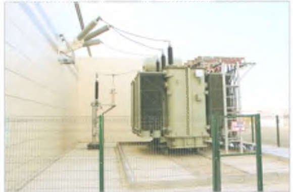
10/35/10 kV-luq güc transformatoru
